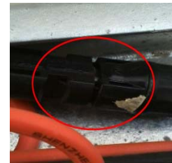
The cable is loose
